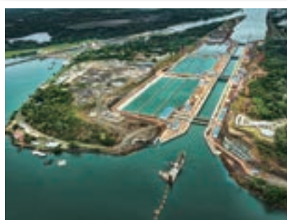
▲ Filling & Emptying System for Panama Canal
